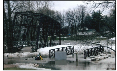
Parshallburg Bridge in Cole Park , off it's base (After the storm)
